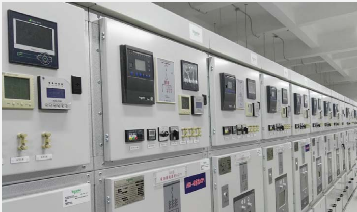
The energy for the data center is distributed over more than 50 switch-gear controlled circuits in the medium and low voltage domains .
